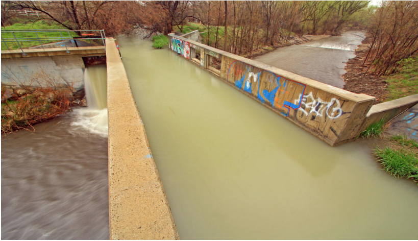
Figure B-2. Jordan and Salt Lake City Canal crossing Little Cottonwood Creek (USGS 2011).
